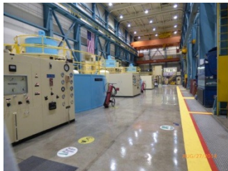
Hydro-Electric Turbine Room
