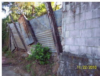
Damaged Retaining Wall
